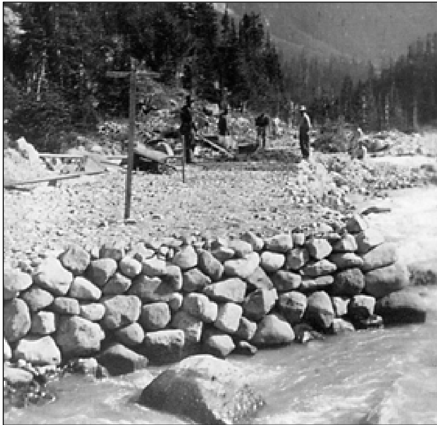
Figure 3.9 White River Road Under Construction above Silver Falls in 1916. (Courtesy Arthur L. Storbo)
